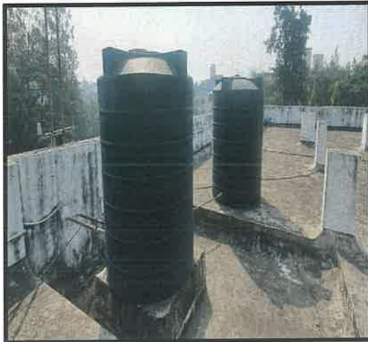
Figure 14: Water tank System
